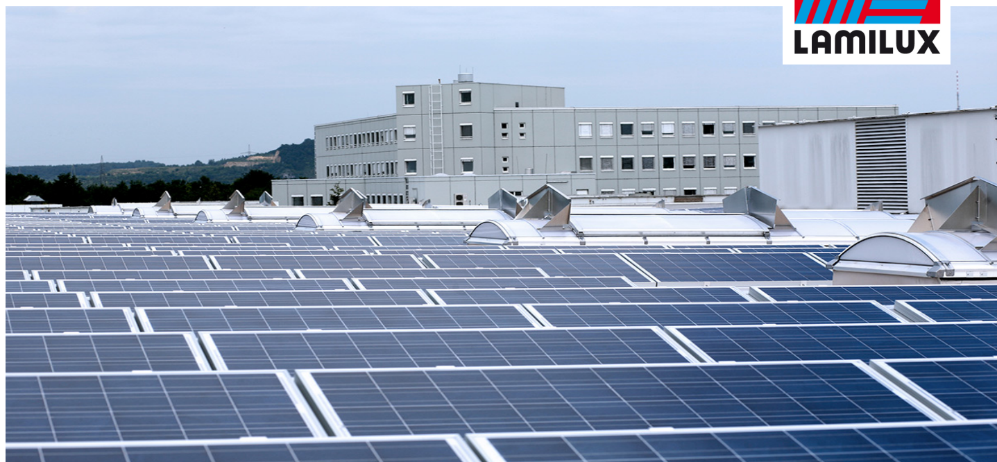
Schneider Electric, Regensburg, Germany
